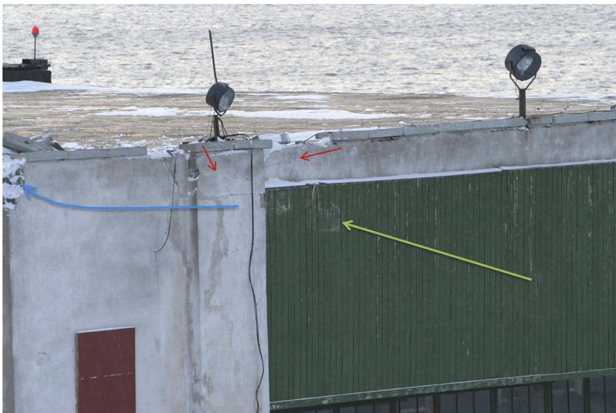
Figure 5: The point of impact on the south (left) corner of the hangar. The green arrow indicates the direction from which the helicopter approached, and the red arrows show blue colour deposited on the concrete. After the impact, the helicopter continued to the left as indicated by the blue arrow.
